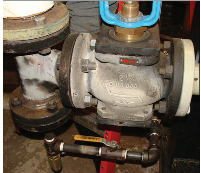
Photo 2: A bare tee and gate valve are part of a steam distribution system in a building's mechanical room; the steam is generated by a central steam plant. Notice how easy it is to identify bare components of pipe distribution systems in mechanical rooms.
