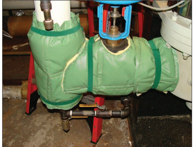
Photo 5: Two components from Photo 2 after being fully insulated using a modular thermal insulation kit.
